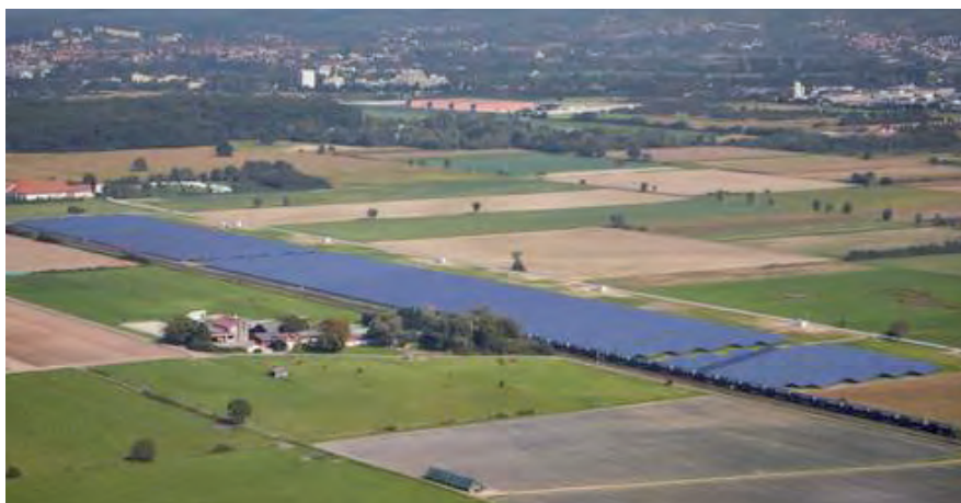
Photovoltaik-Anlage in Hohberg (©ADSOBA GmbH)
